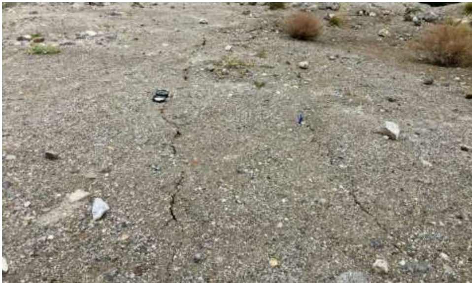
Photo 8-20 Development of Parallel Joints near SCO Building.
