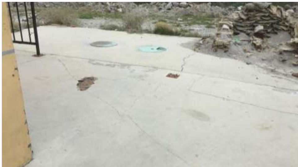
Photo 8-16 View of Recently Generated Joints between Tunnel-2 & 3.
